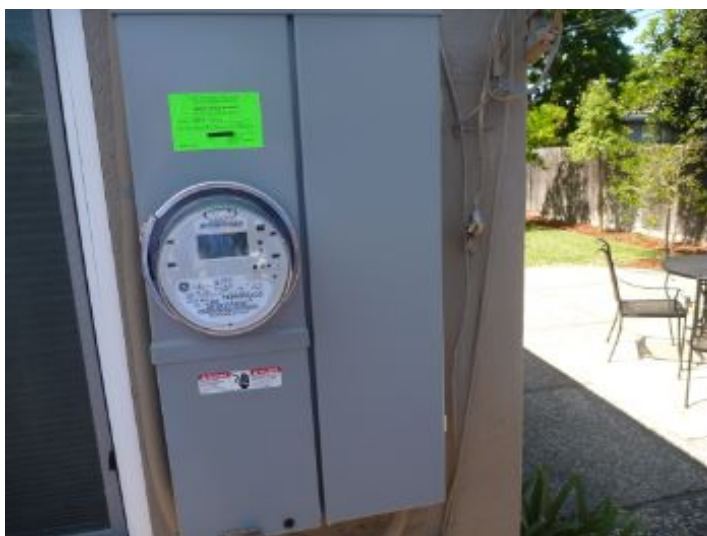
New electrical panel
